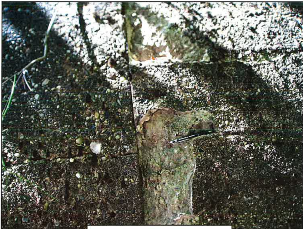
#8. Spalling of Concrete on Dam
