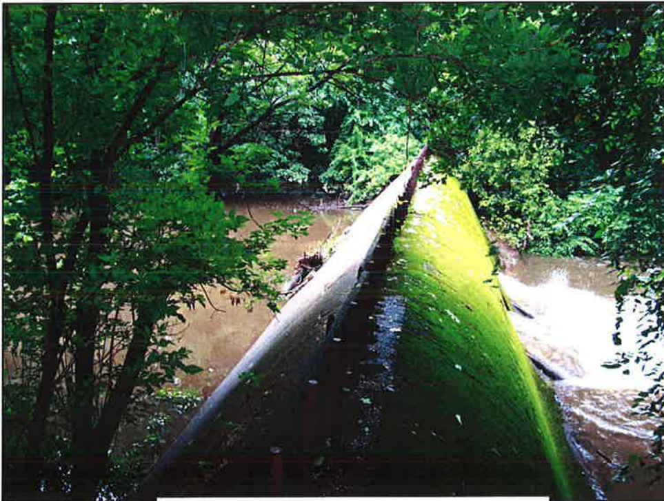
#2. Moss on Dam – Debris on Conduit
