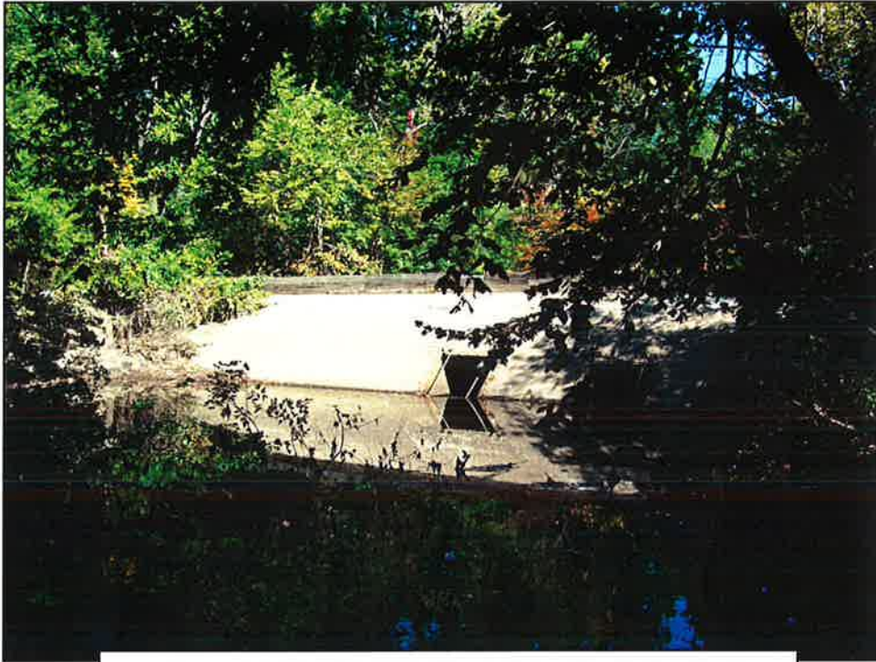
#5. Dam with Overhanging Trees from the Embankment
